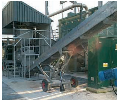
Compact plant area
